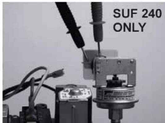
Low gas pressure switch
