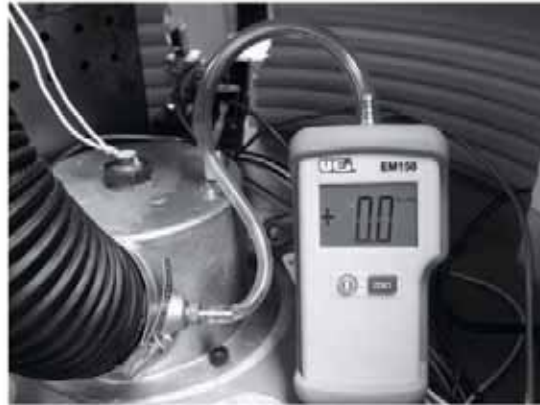
Blower prover and blocked outlet pressure
