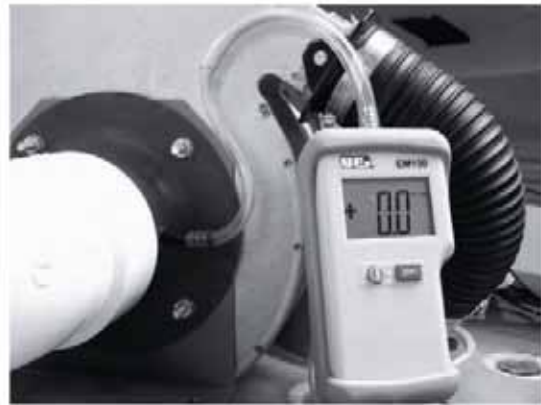
Blower inlet pressure
