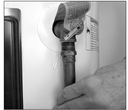
Figure 15 - The T&P Relief Valve discharge pipe must be installed properly and piped to an adequate drain.
